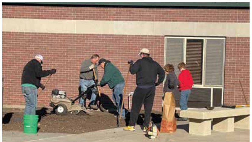
Members of the Grounds Ministry working to clear the existing trees, bushes and rocks in preparation for the spring planting season
